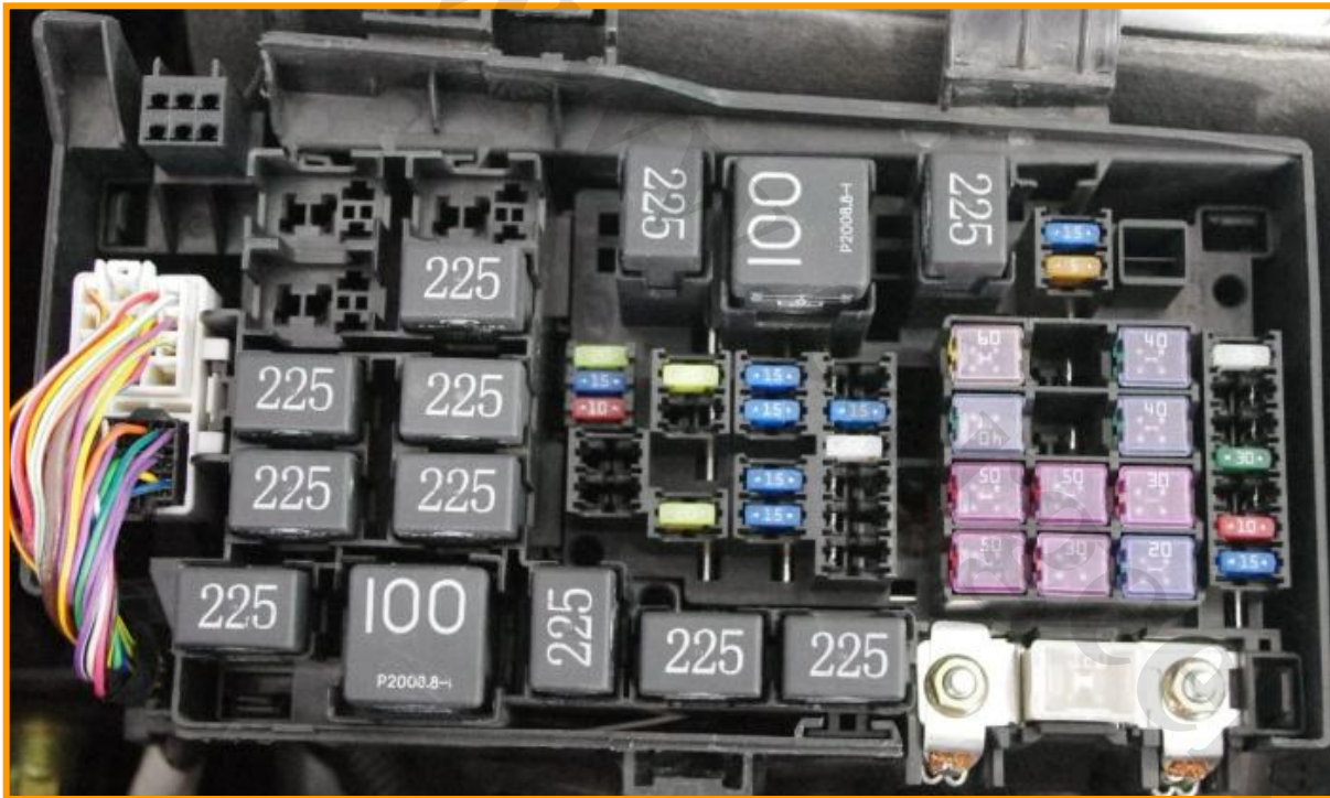
Front hood fuse and relay box
