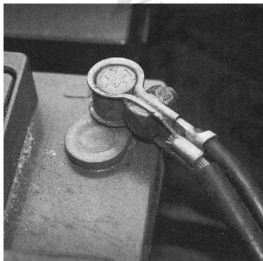
Figure 9.61 Battery earth connection – so easy to forget the obvious
